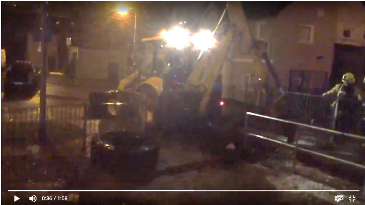
Photo 6.1: JCB removing a large tractor tyre trapped at the pedestrian bridge in Orchard Court in March 2013.
