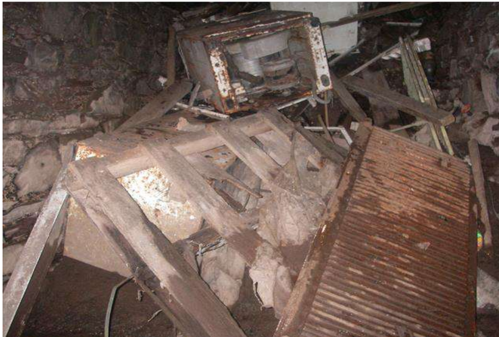
Photo 4.4: Above photo washing machines, radiators and wooden pallets trapped in the underground culvert.
