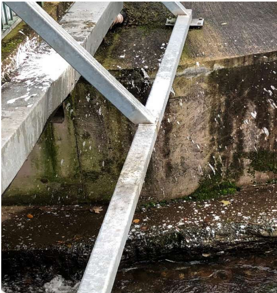
Paint disposed of by being dumped into the River Bride
