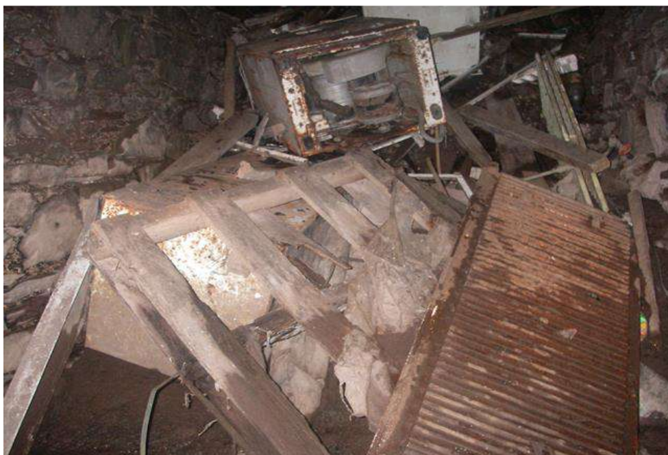
Photo 4.4: Above photo washing machines, radiators and wooden pallets trapped in the underground culvert.
