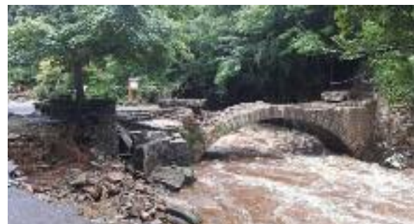
Figure 15. Old Mill Bridge in Buncrana, County Donegal, was also destroyed in the floods caused by heavy precipitation in August 2017 (Maguire, 2017)
