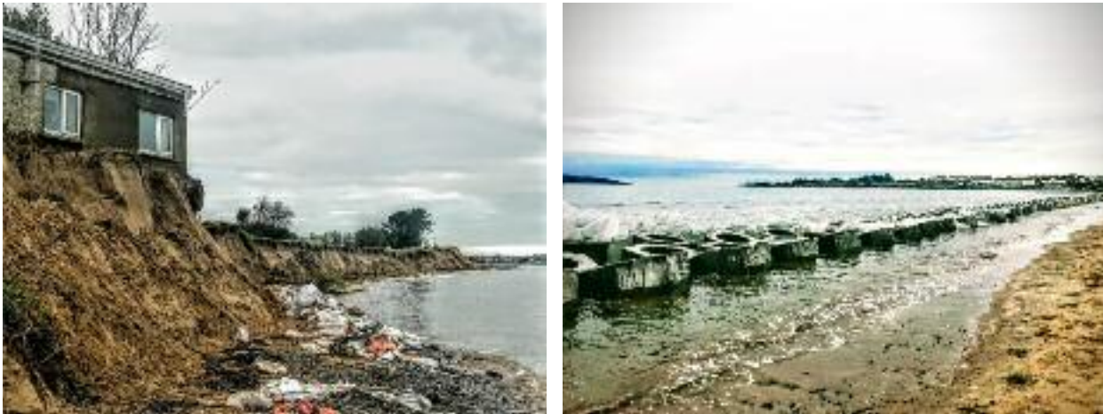
Figure 9. Dwellings in Portraine on the brink of falling into the sea because of coastal erosion (left); €500,000 worth of concrete blocks installed as a short-term solution to coastal erosion in Portraine (right) (Comerford, 2018)
