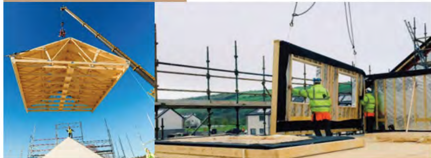
Figure 8 Offsite light timber frame construction (Photo credit: Derome AB, SE and Cygnum, IE)
