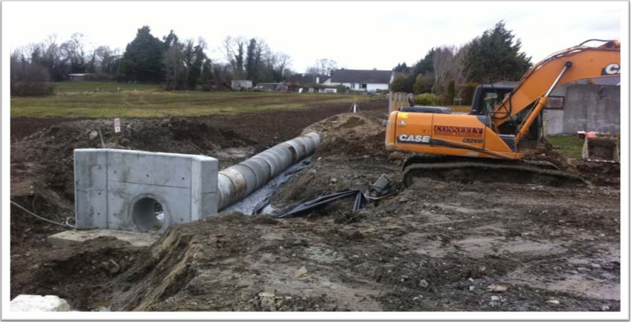
Photo of North East Bund, drain is culverted and headwall and bund under construction in foreground
