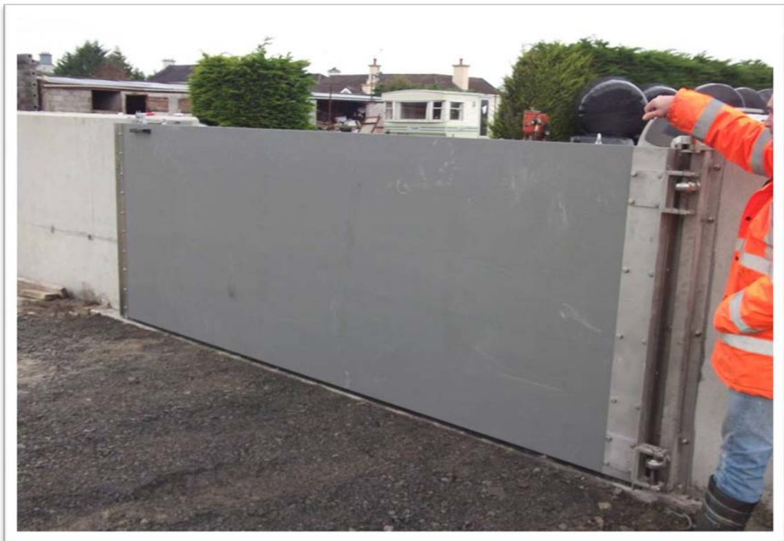
Flood gates in place
