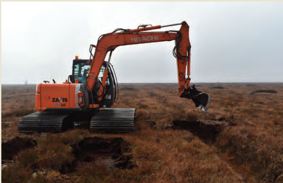
Peat dams being placed into a drain by 'The Living Bog', blocking the drain to keep water on the raised bog. For more information go to http://raisedbogs.ie/
