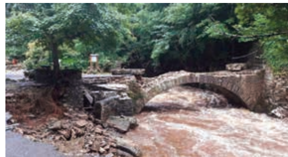
Figure 15. Old Mill Bridge in Buncrana, County Donegal, was also destroyed in the floods caused by heavy precipitation in August 2017 (Maguire, 2017)
