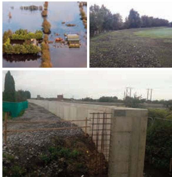
Figure 14. Flooding near Athlone town along the River Shannon (left) (Fitzsimons, 2018); implementation of a flood embankment (right) and flood-defence wall (below) on Brick Island in Athlone (Athlone Flood Alleviation Scheme Project Team, 2019)
