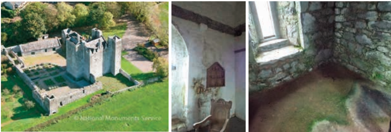
Figure 25. Aerial view of Barryscourt Castle, County Cork (left) (DCHG); mould growth on the interior of the castle (centre and right) (OPW)
