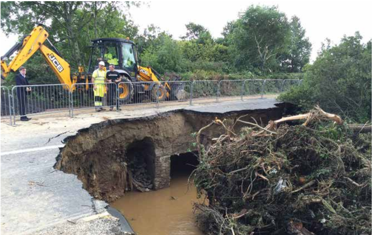
Figure 3.3: Damage to the R328 Derry to Moville Road in Co. Donegal caused by pluvial flooding during ex-Hurricane Gert, August 2017. Source: Brian Hutton/PA.
