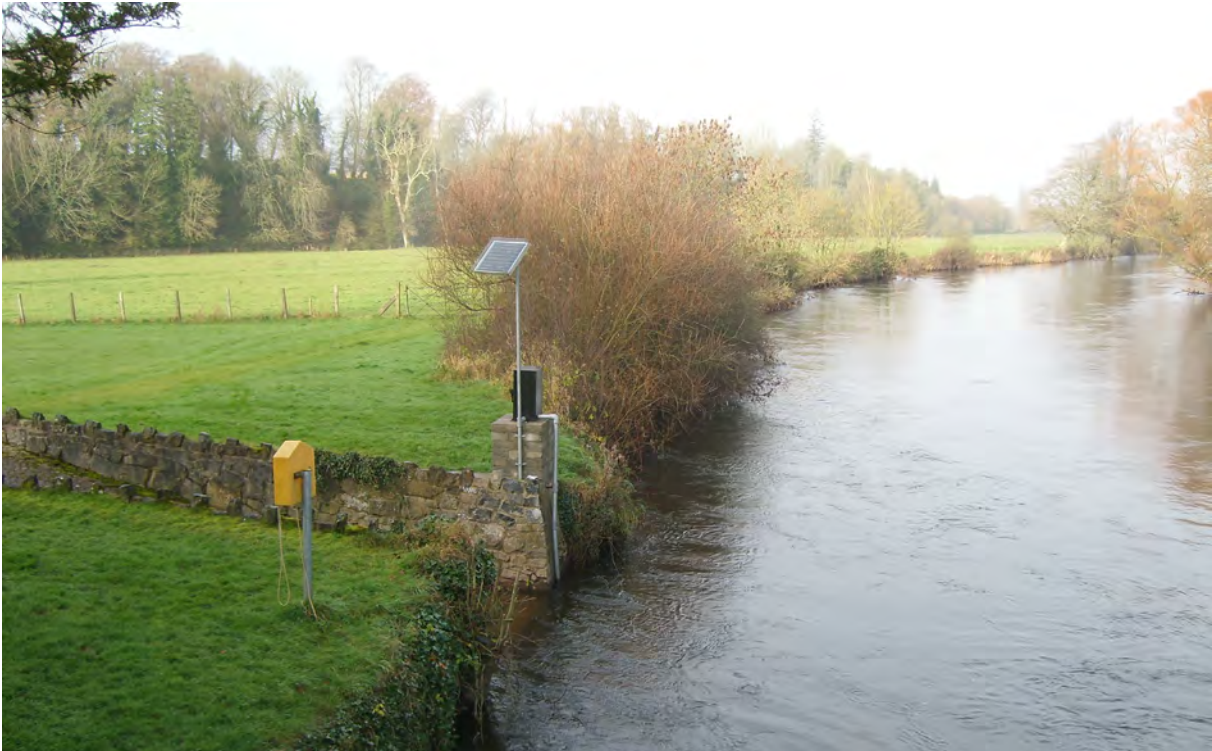
Figure 1-3: River Gauge with telemetry
