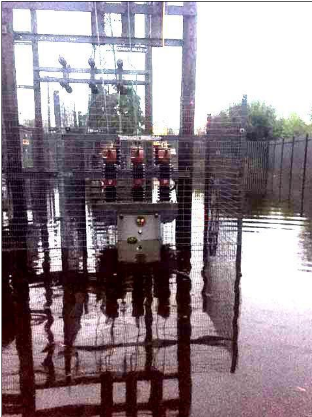
Figure 7 Flooding in an outdoor HV Station
