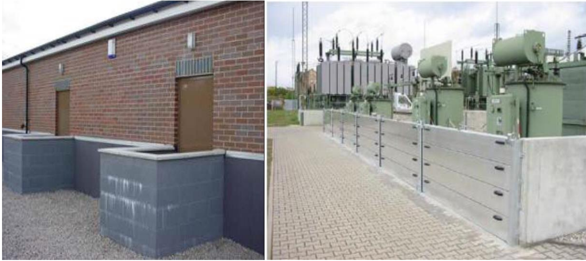
Figure 12 Bunding of Control Buildings Figure 13 - Bunding of Electrical Equipment
