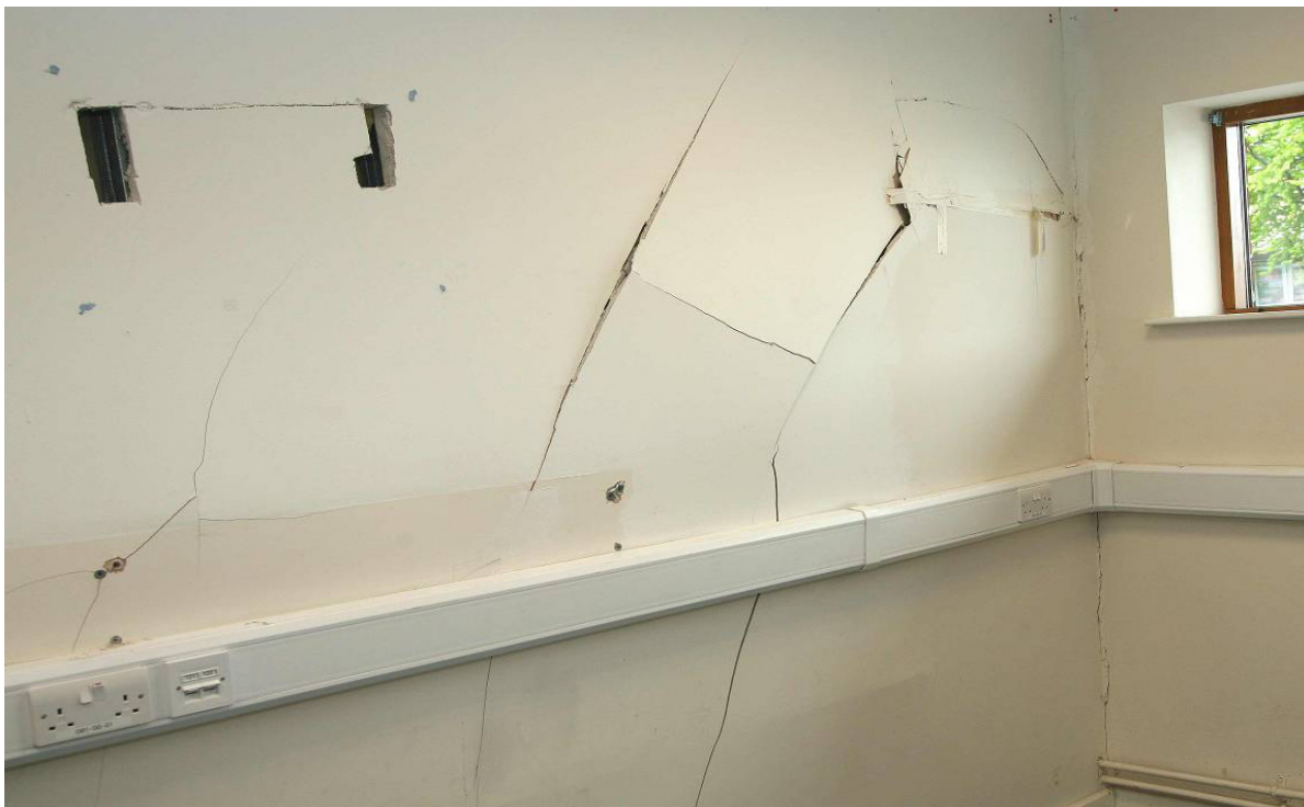
(viii) Bulging of wall finishes
