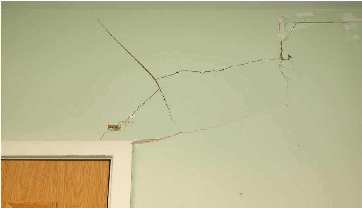
(iv) Cracking at head of door
