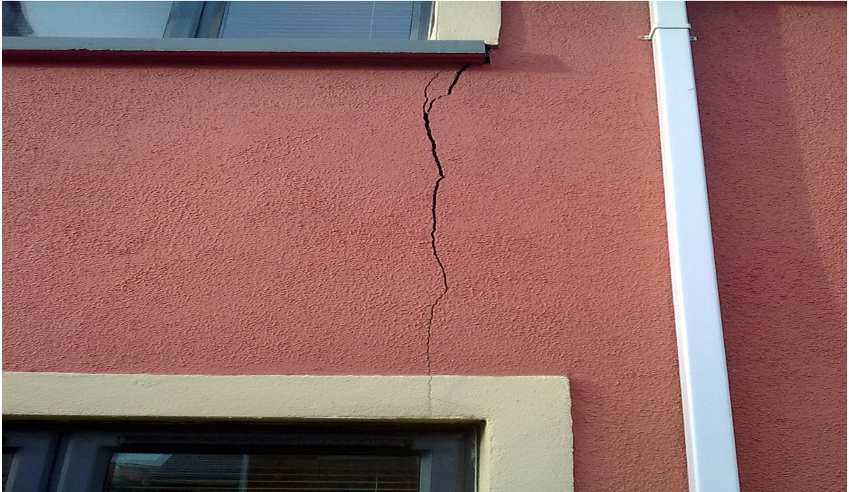
(ix) External wall cracking
