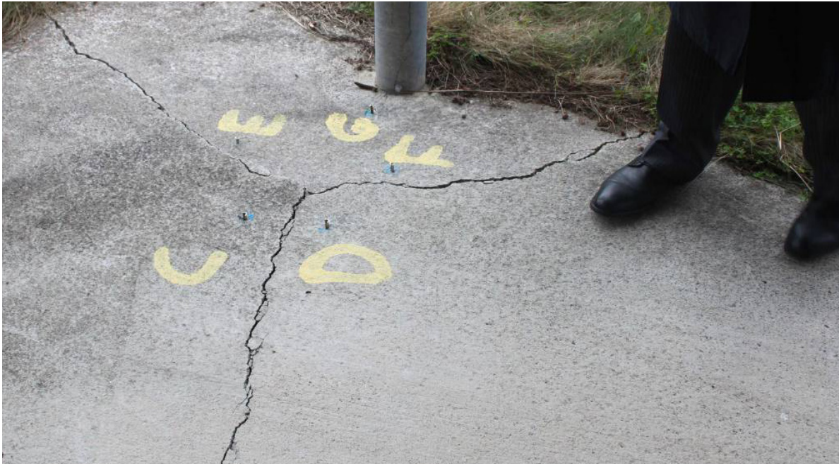
(ii) Cracking of footpath
