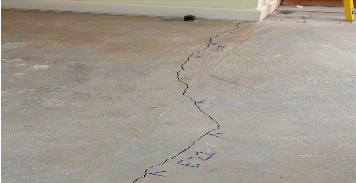
(i) Cracking of floor slab
