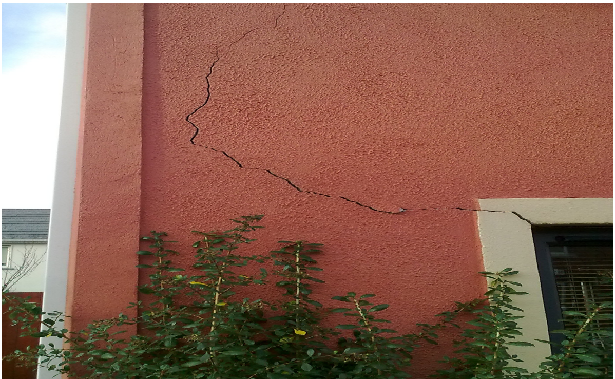
(x) External wall cracking
