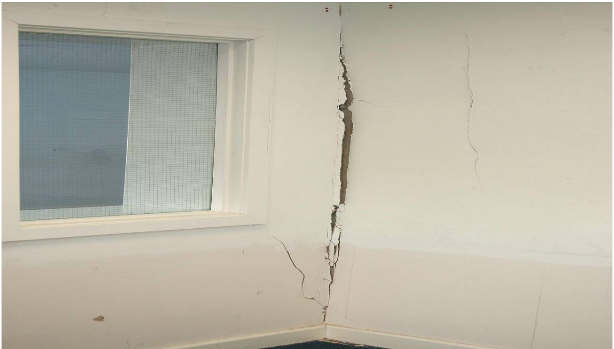
(vi) Bulging of wall finishes
