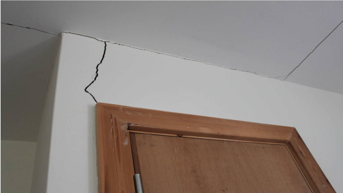
(iii) Cracking at door frames
