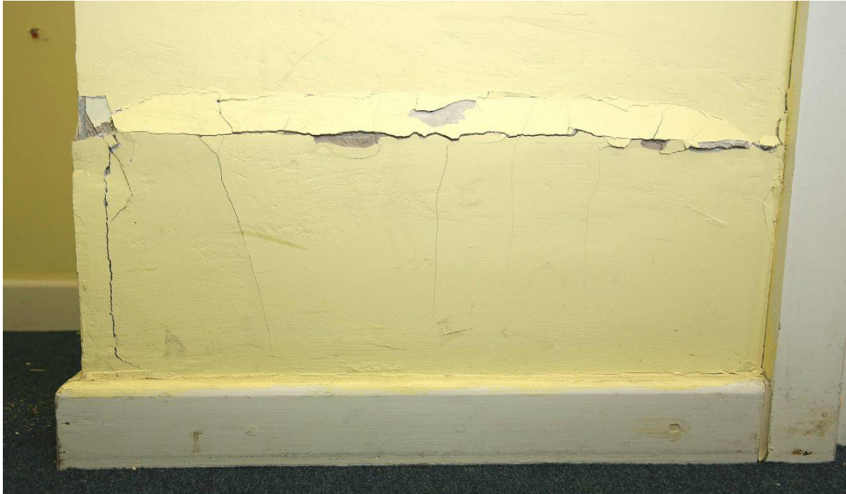
(vii) Bulging of wall finishes
