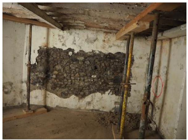
P36.6 Portion of a basement wall exposed to reveal the alluvial and esker stones of which it is made.
