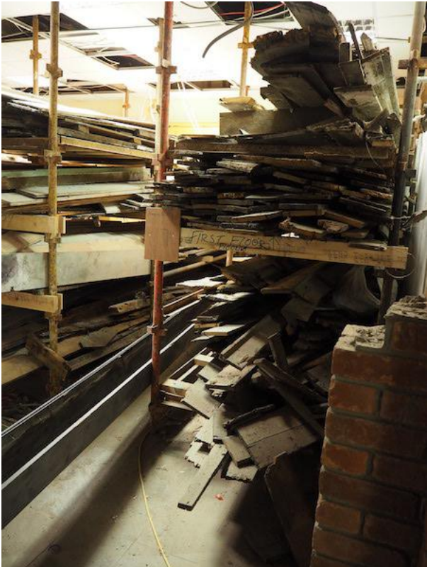
P42.1 Removed material is stored in racks, organised by building and by floor
