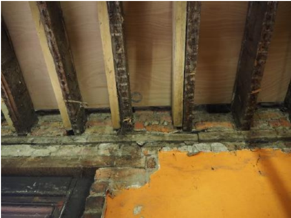
P15.5 The masonry surround joist ends is precarious
