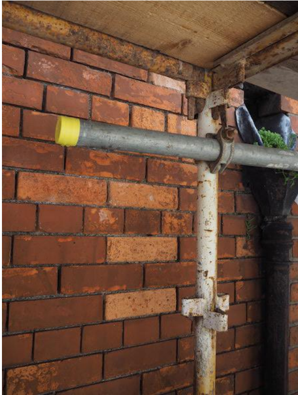
P6.1 Many bricks have lost their protective 'fire-skin', leaving them prone to more rapid decay
