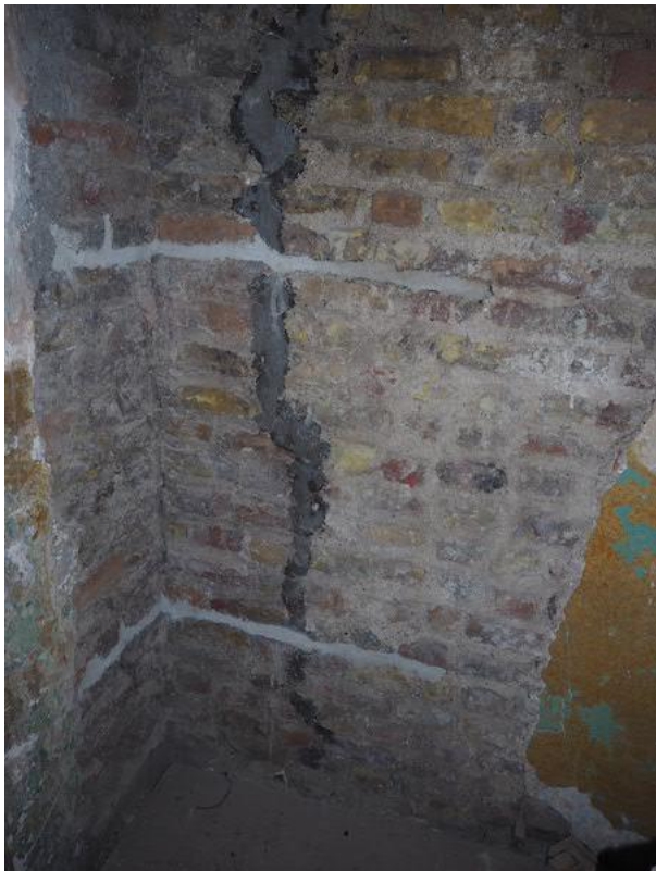
P17.5 Stainless steel helibars inserted to tie the facades to flanking walls
