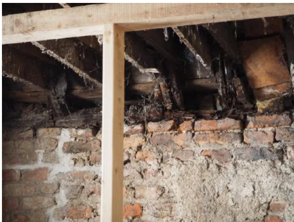
P16.5 Timber decay at roof level
