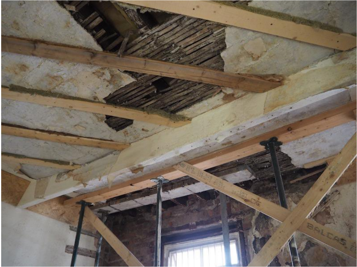
P29.1 The diagonal planks on the ceiling are an older attempt to retain the decayed plaster ceiling in position: it is probably beyond repair.
