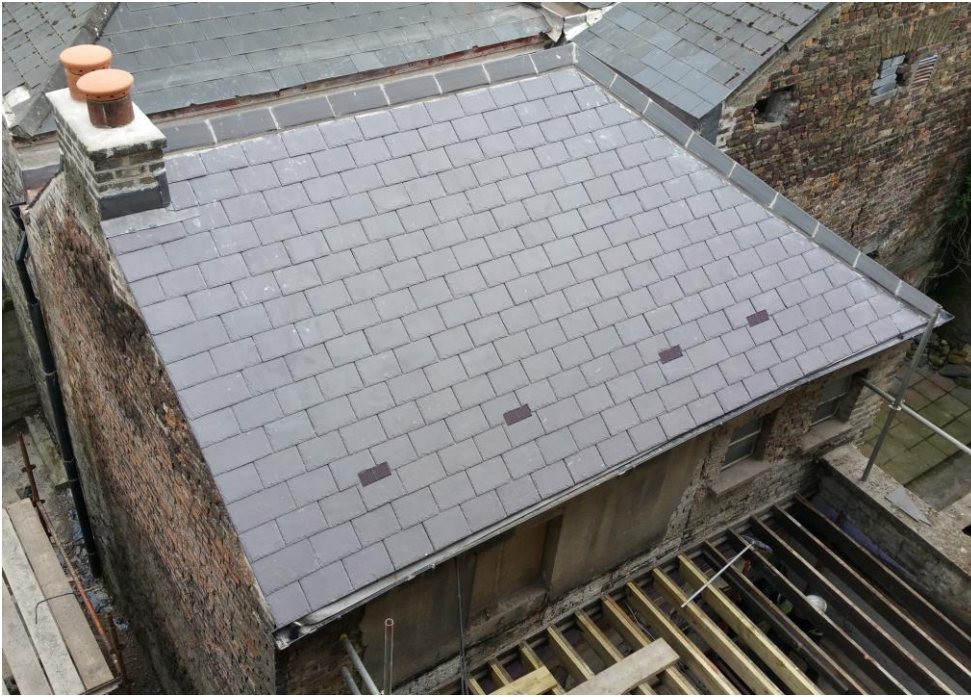
Completed roof of building at rear of no. 14 and temporary works on flat roof (Photo: P. Walsh)
