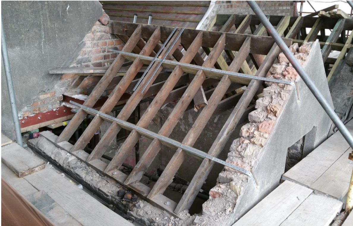
Steel beam (dark red) and steel ties in place in no. 16 (Photo: P. Walsh)
