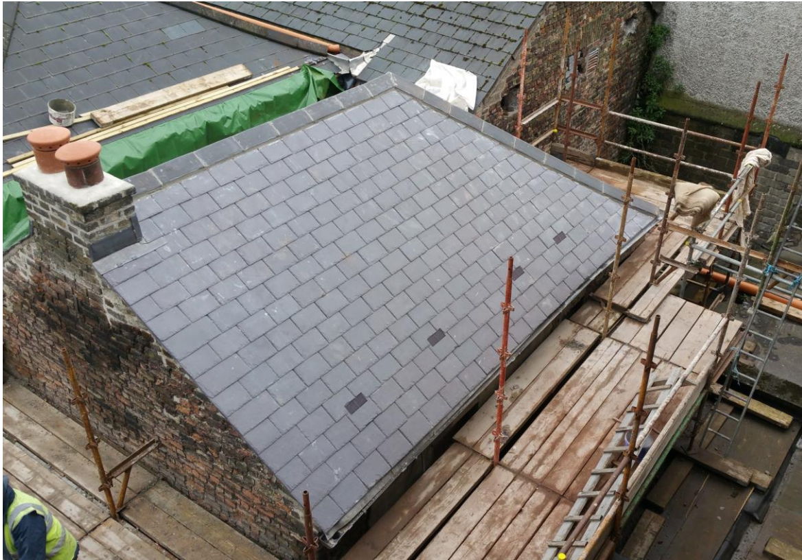
Roof of building at rear of no. 14 near completion (Photo: P. Walsh)
