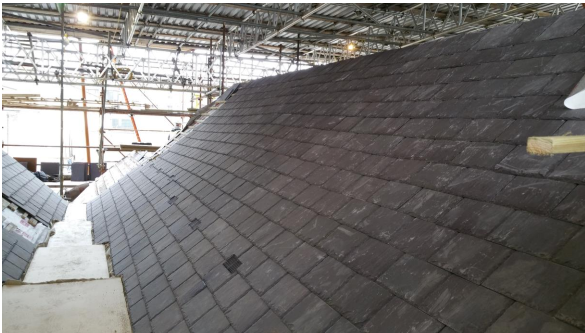
Slating in progress on nos. 15, 16. Note vents in place (Photo: P. Walsh)
