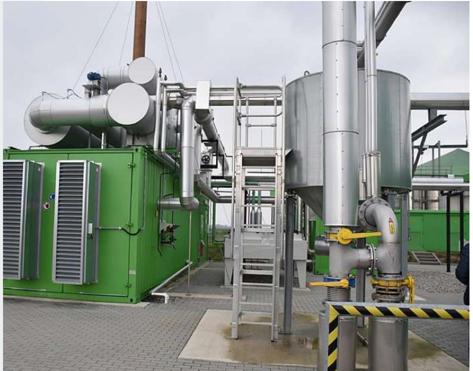
Image: CHP Engine on a biogas plant (Schwedt)
