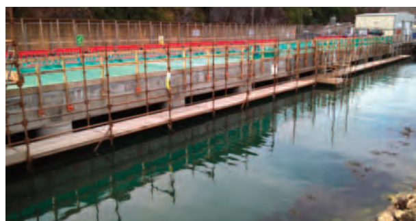
West Wharf Remedial Works Phase 4, Dunmore East FHC Construction Contract Works in progress 2019
